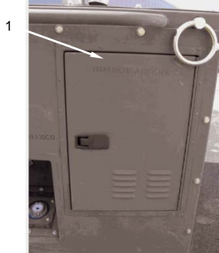
Figure 25. Burner Access Door.
