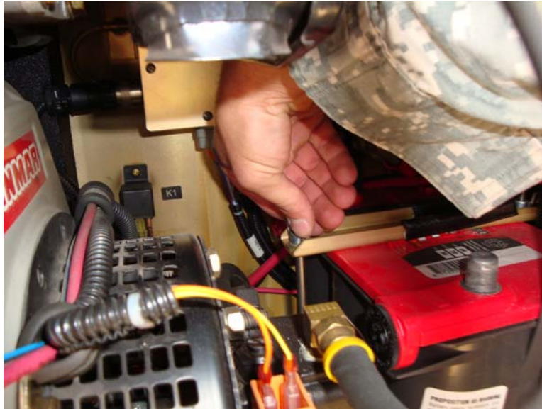
Figure 7. Remove Hardware Securing Battery T-bar Farthest from Access Door.
