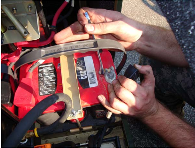
Figure 52. Install Negative Terminal on Battery Closest to Access Door.
