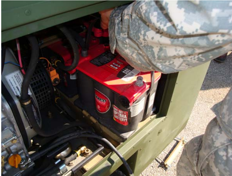
Figure 26. Install Battery Closest to Access Door.
