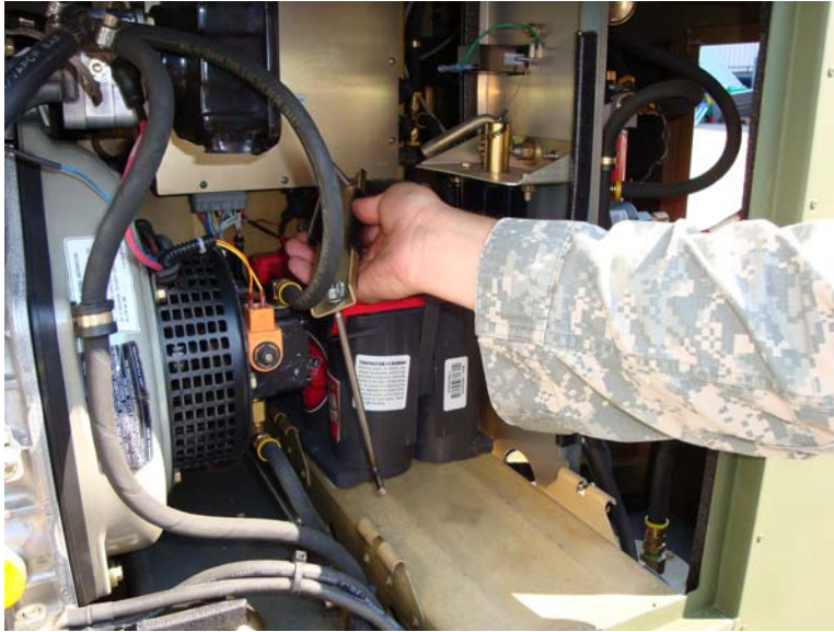
Figure 8. Remove Battery Hold-down Bracket of Battery Farthest from Access Door.
