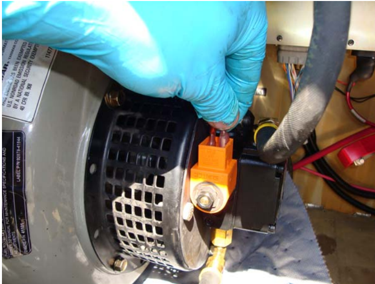
Figure 22. Reconnect Wires to Burner Fuel Pump.
