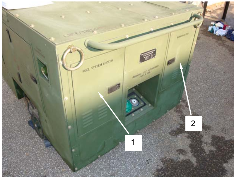
Figure 9. Closing Fuel System and Burner Access Doors.
