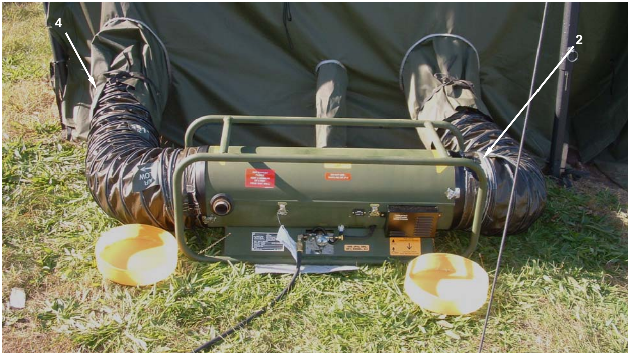
Figure 6. SHC-60K Heater Exchange Process.
