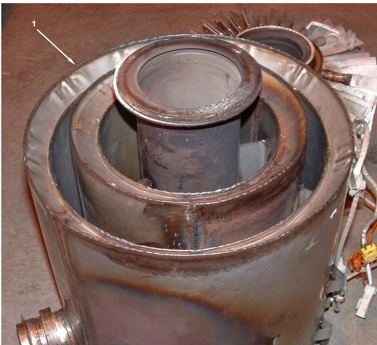
Figure 3. Clean the Heat Exchanger Assembly.
