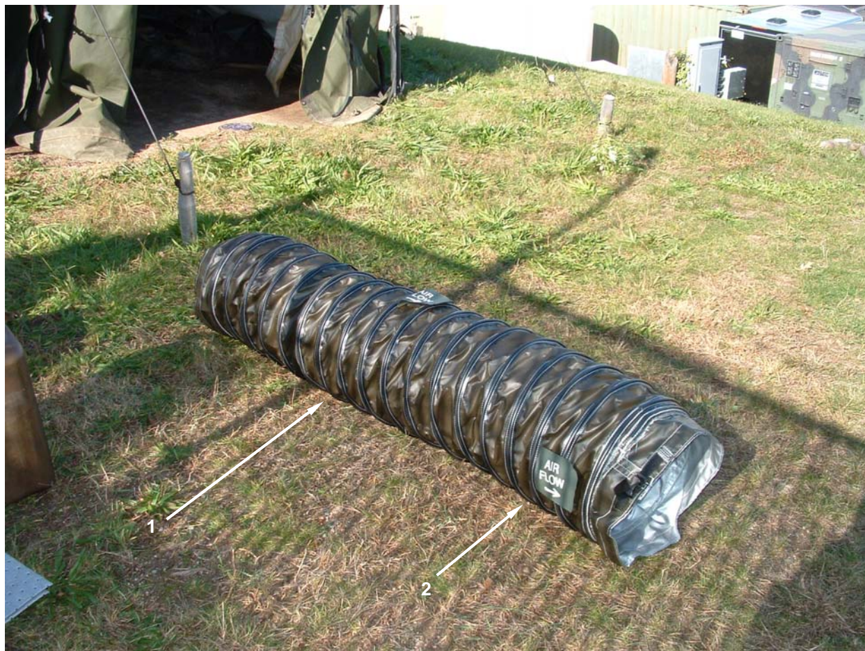
Figure 18. Air Supply and Return Ducts.
