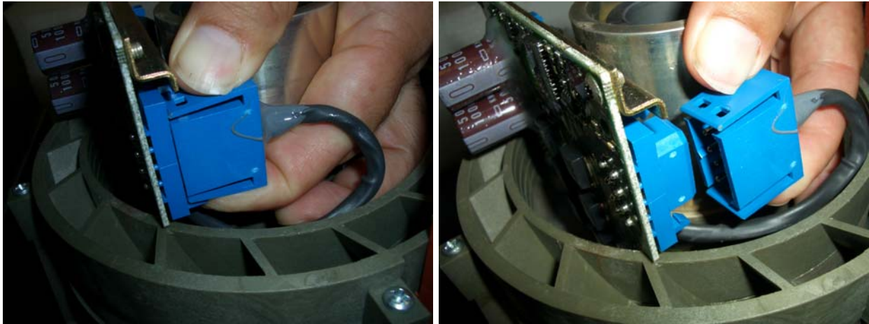
Figure 5.6-21 Detail, Removal of Printed Circuit Board Connector
